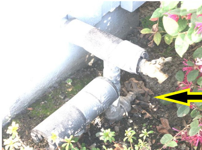
HOUSEHOLD MAIN WATER SHUT OFF VALVE
